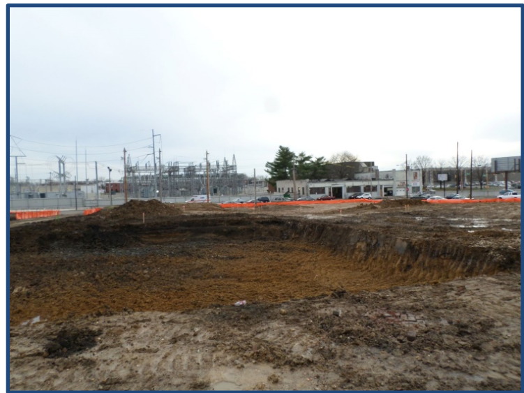
This photograph shows the initial excavation under the former Laycock Clutch building after the slab was removed.
