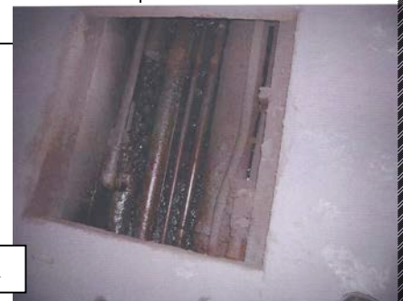
Pipes in the trough
