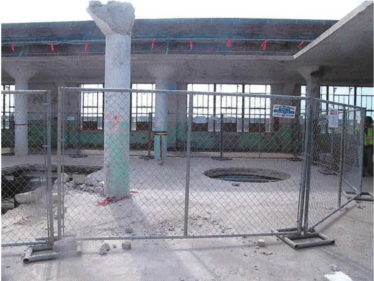
Photo 1 of 1: Floor openings where debris was removed from the site
