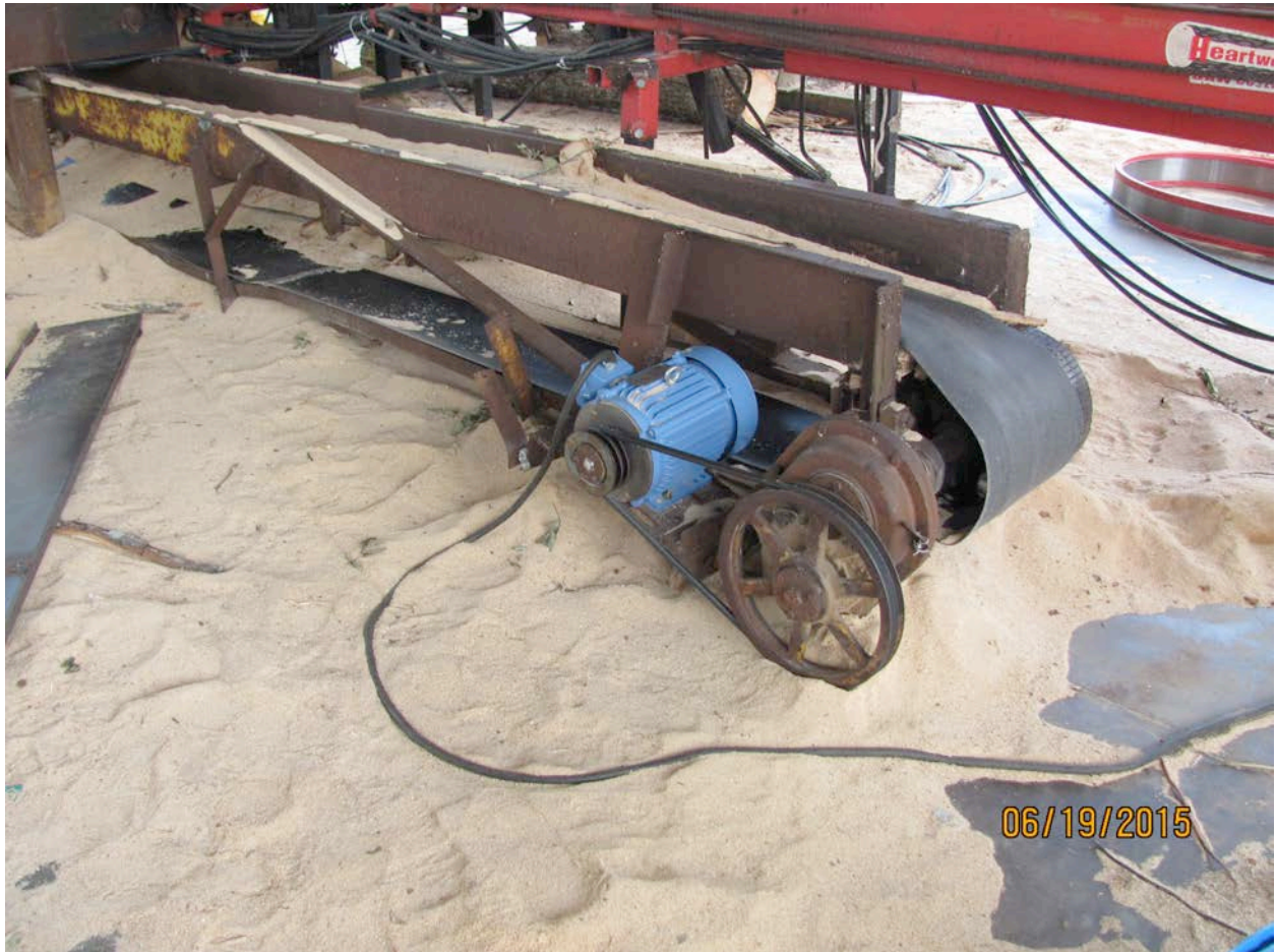
Photo 2 of 2 – The photograph shows the flexible cord run across the concrete floor at the mill and it was not protected from damage.
