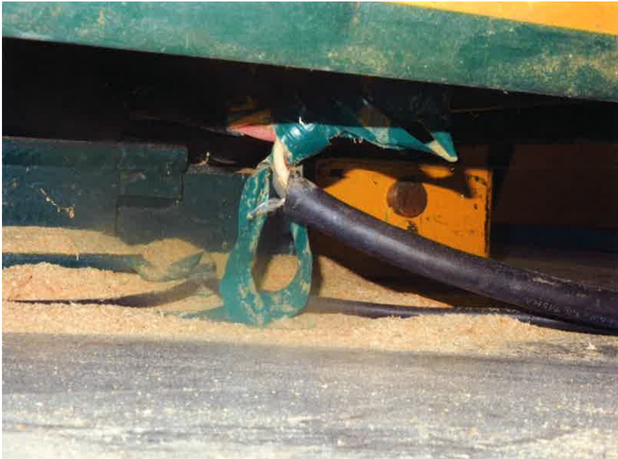
Photo 2 of 2 – Photo shows the power cord for the lifting table and one of the several splices to the cord.
