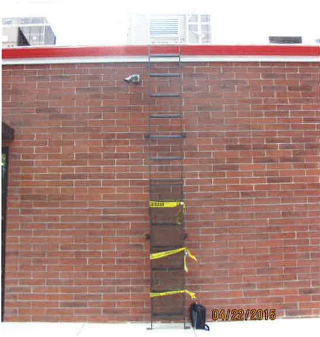
Photo 1 of 2 – This photo shows the fixed ladder bolted to the building for roof access.
