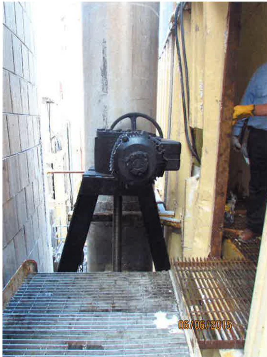
Photo 1 of 2 – This photo shows the view of the valve and the unguarded holes between the platforms and building surfaces.
