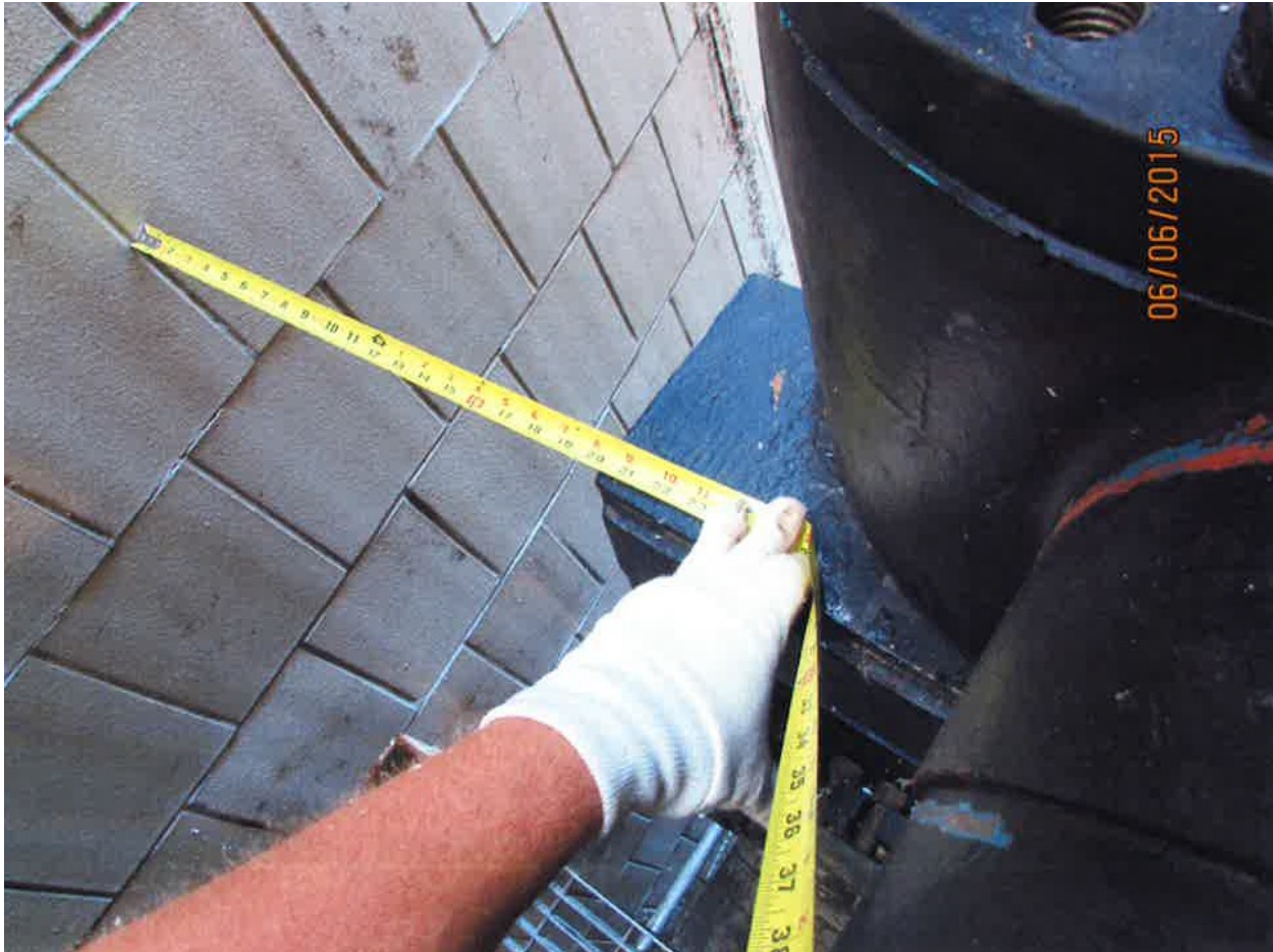
Photo 2 of 2 – This photo shows the view of the valve and the unguarded 20 inch hole between the valve and building wall.
