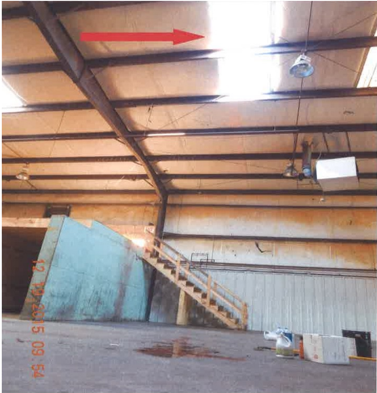
Photo 1 of 2 – Photo of shows the inside of the building which was in process of having its roof replaced. The victim was working near an opening on the roof when he slipped and fell.
