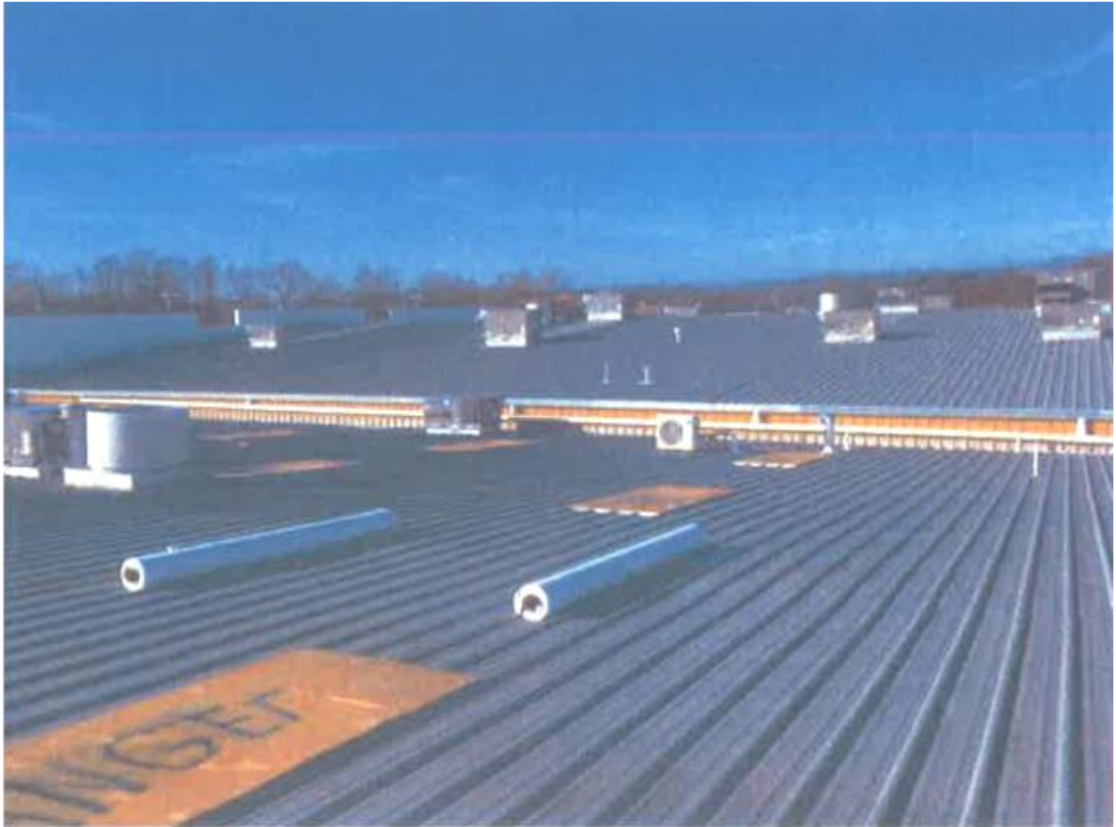
Photo 1 of 1 – The skylights were covered following the incident.
