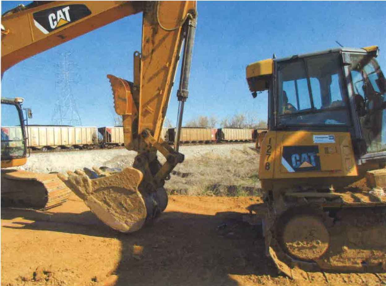
Photo 1 of 1 – View of the bucket of the excavator and the dozer. The victim was crushed between the bucket and the rear of the dozer.
