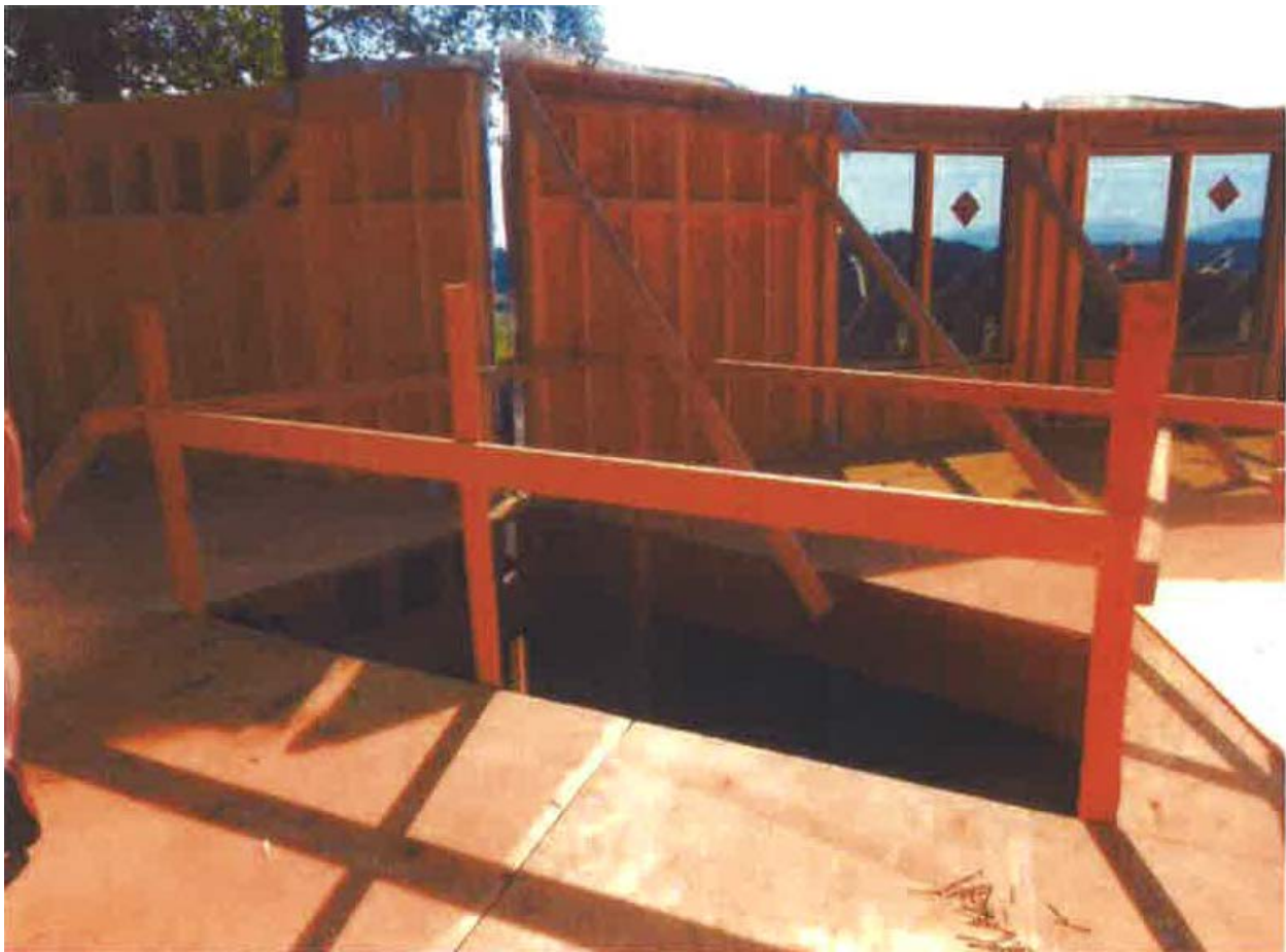
Photo 1 of 1 – Floor opening located on the main living area or center section of the home. The guardrail was not in place prior to the incident.
