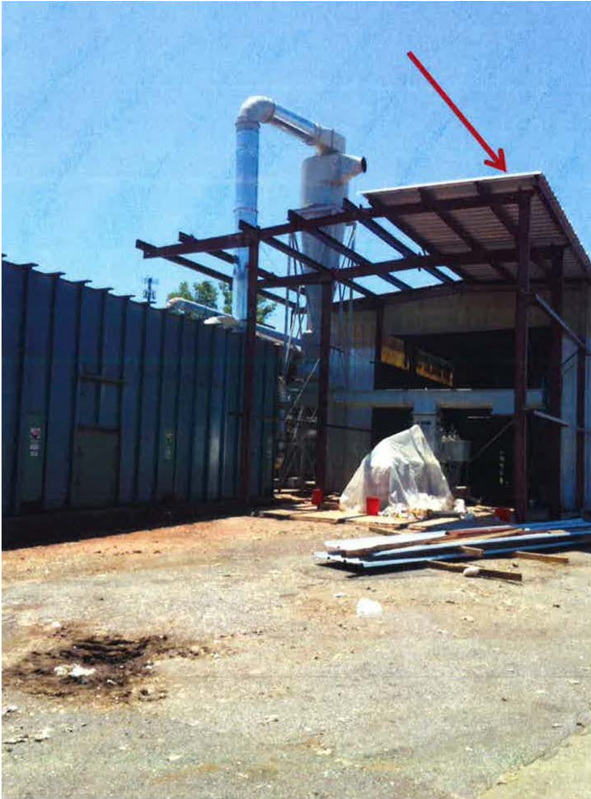
Photo 1 of 1 – Northeast corner of the roof designated by the red arrow where the victim stepped off the roof falling approximately 24 feet.
