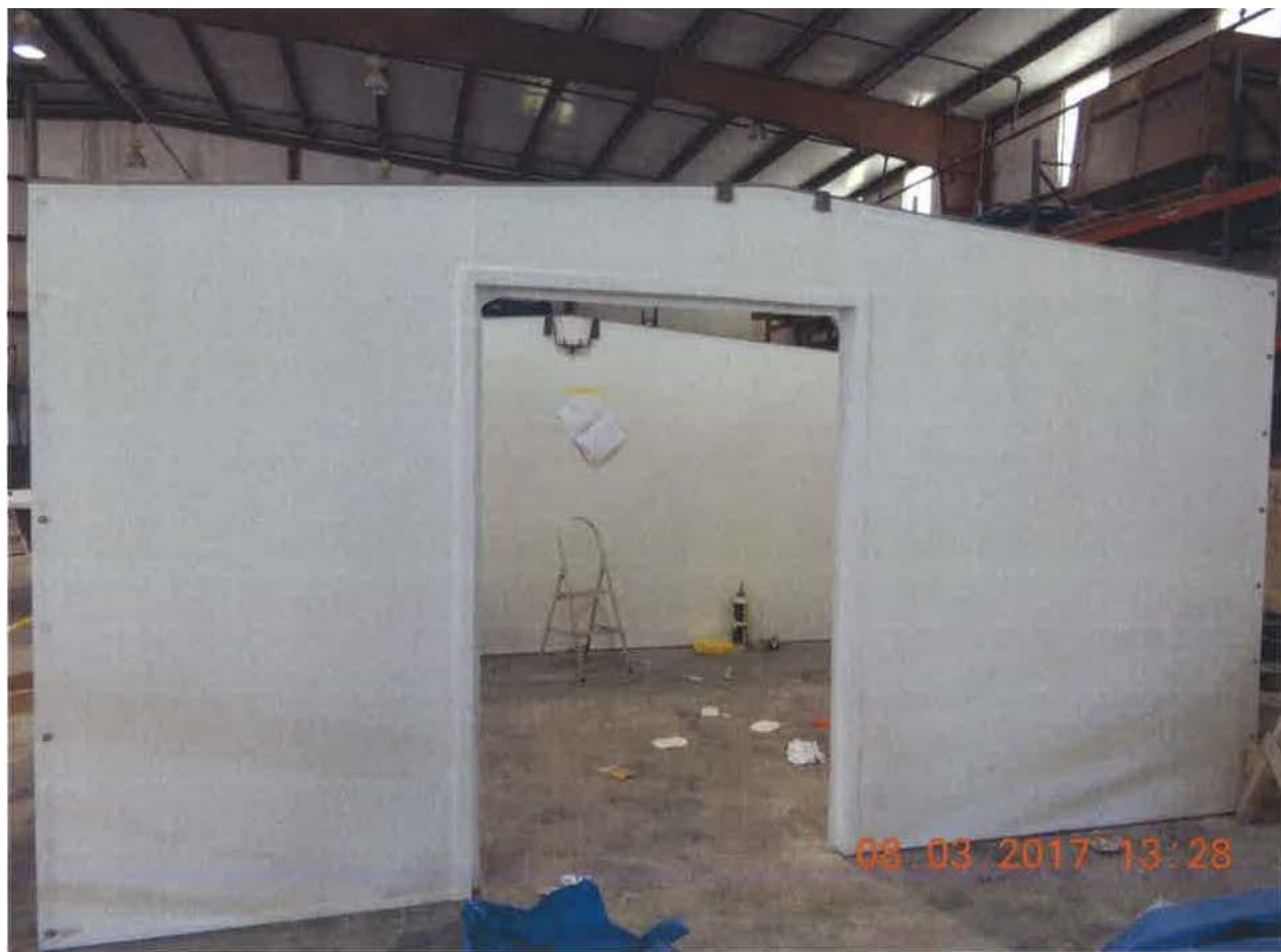
Photo 1 of 1 – The bracket is shown above the step stool where the victim tried to lift the interior beam into place.
