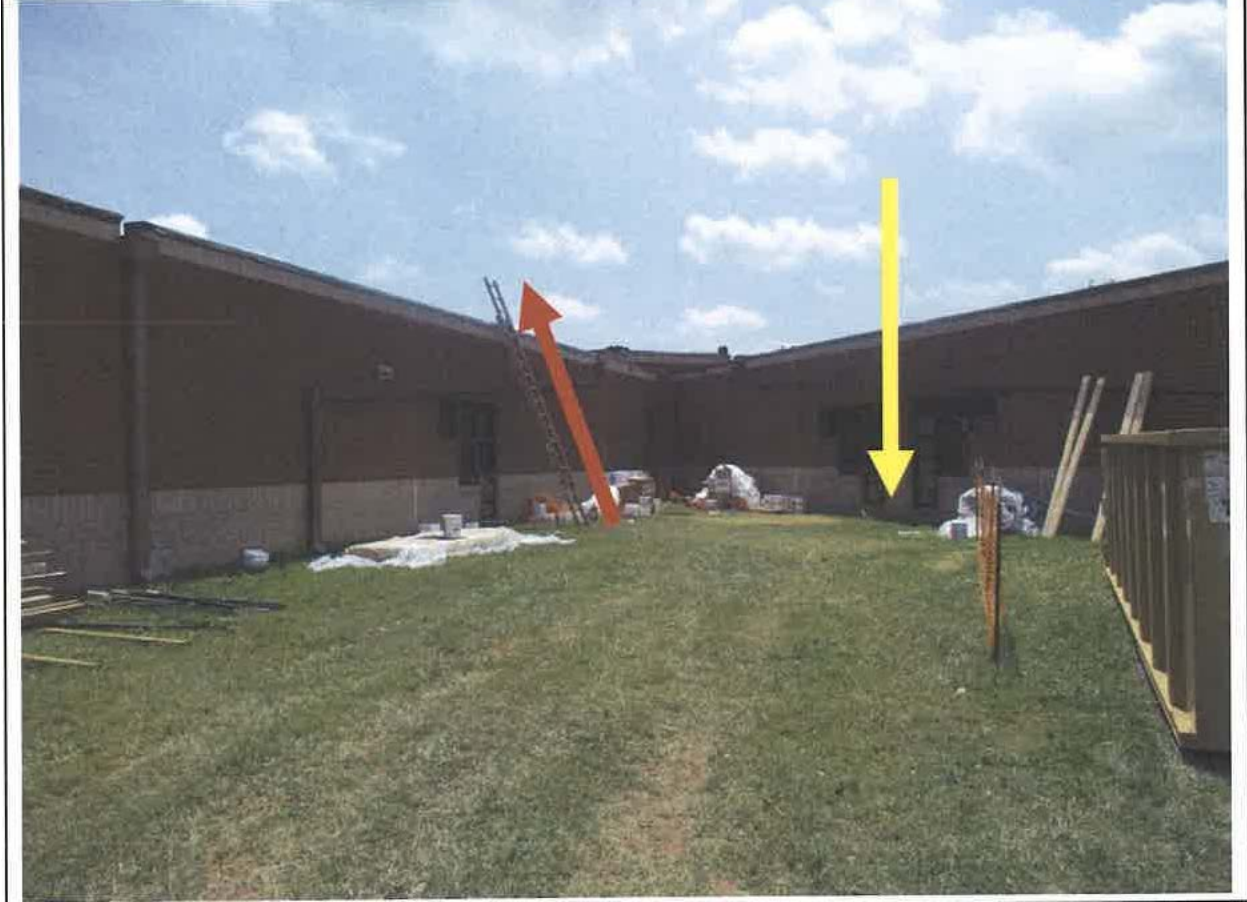
11 Fall from elevation (roof)--Inspection #1410206 Ragan Construction
