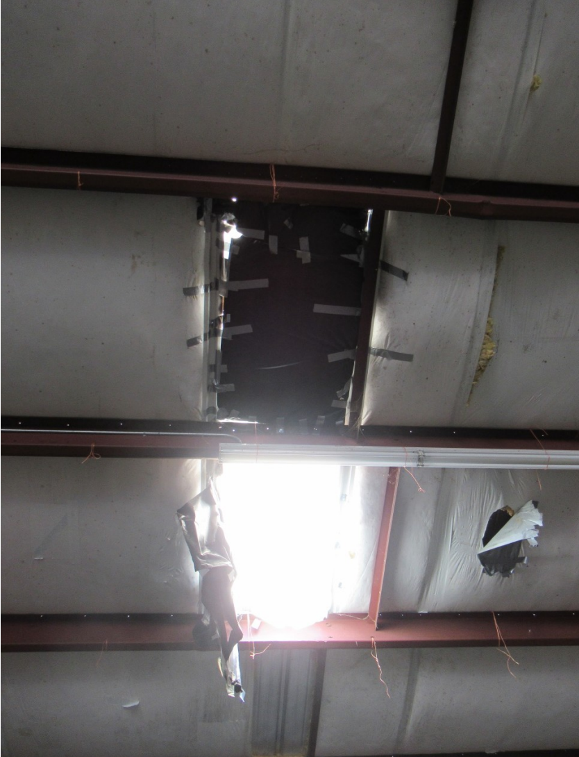
6 Fall through skylight--Inspection #1472242 John Hurd
